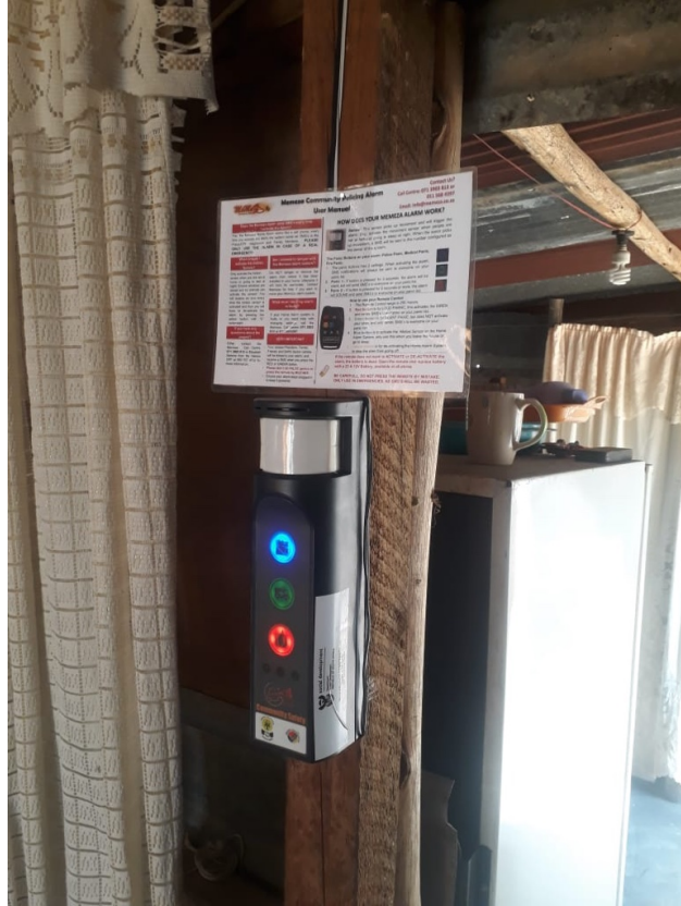
Figure 10: The Police Alarm System
